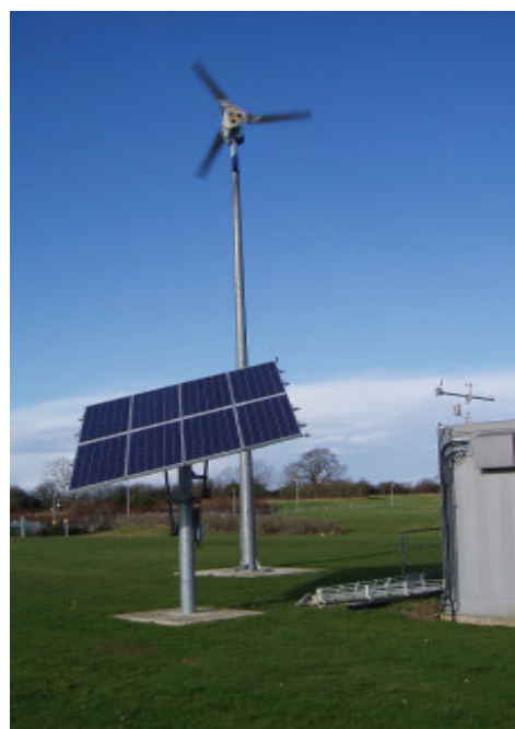
Solar array and wind turbine powering a BTS at Swindon test site
